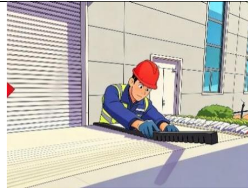
Place upper EVA strips on modules, one gap holds two modules per EVA strip
